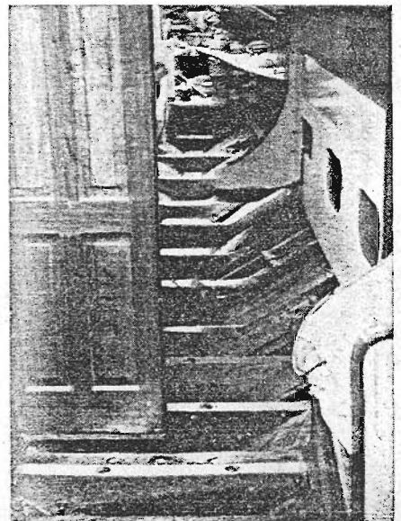
Rotting floors caused Cockatoo II's keel to rock slightly. Solution was installation of eight bronze sister floors, Monel fastened.
